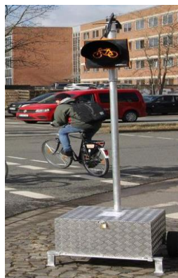
Figure 50. Example of the amber light (option 1). Bike pictogram will be replaced with train.
