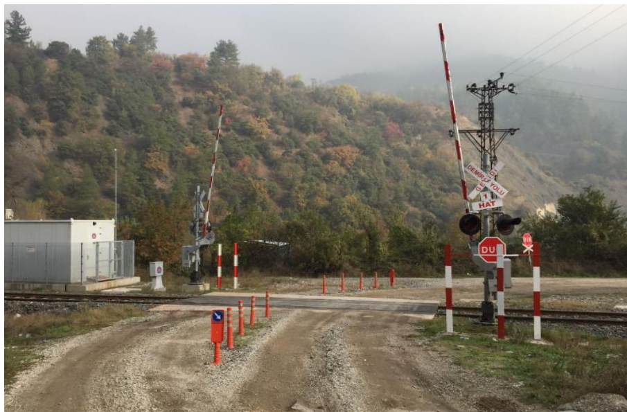
Figure 68. Implementation site 2 Flashing Lights on the Barriers.
