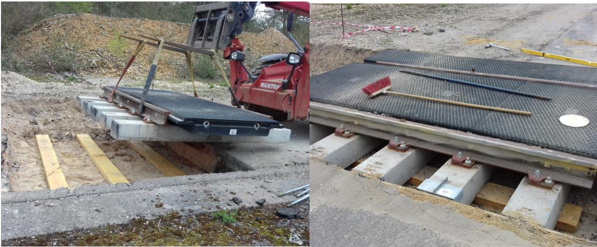
Figure 39. Configuration1 – Bump with wood beams
