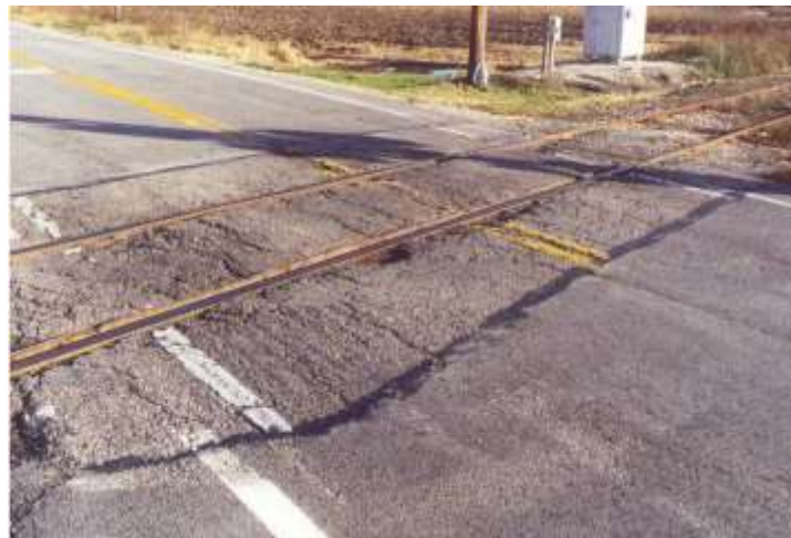
Figure 7 : Potholes asphalt crossing surface
